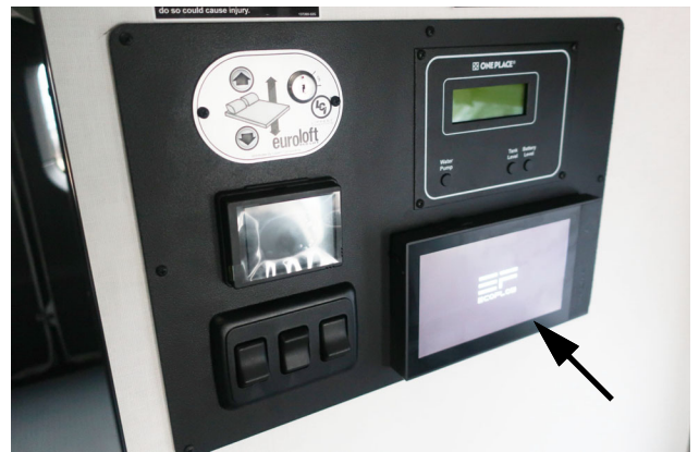
Solar Charge Controller operated through EcoFlow panel. (Located on the monitor panel). -Typical View
