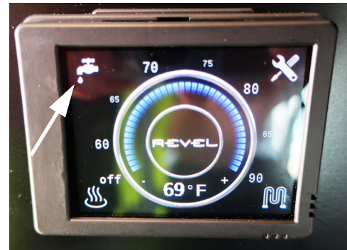
Water heater controls on Systems Monitor Panel -Typical view
