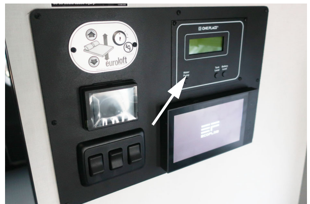
Water pump switch location on Systems Monitor Panel -Typical view
