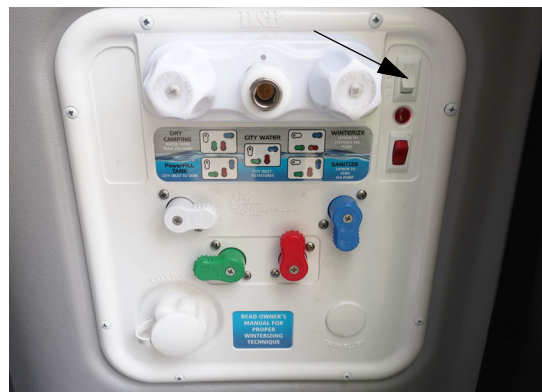
Pump switch -Typical View
