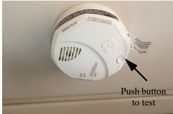
Smoke/carbon monoxide alarm. -Typical View
