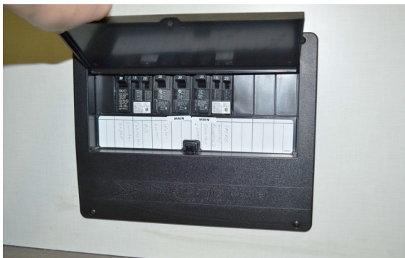
120-Volt Circuit Breakers -Typical View
