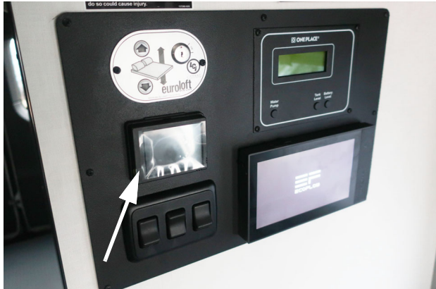
LCD Panel (Located near monitor panel) -Typical View
