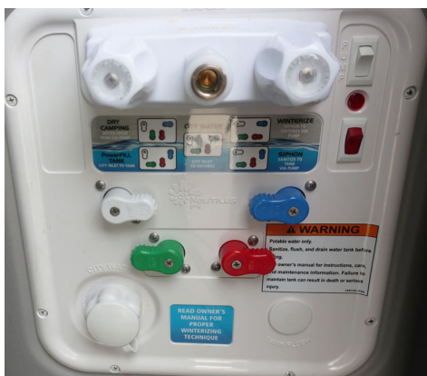
Water Center Panel in “Winterize” configuration (Panel located behind passenger rear door). -Typical view
