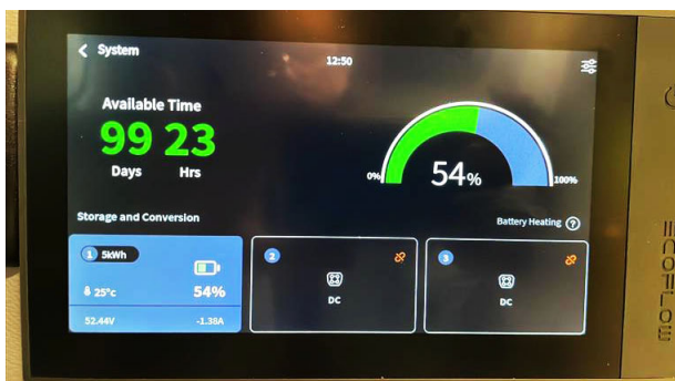
Selecting the System from the main menu will display available time, battery charging/discharging, battery state of charge (SoC) percentage, and temperature. -Typical View
