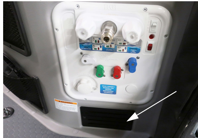
Water Pump (Located below Water Center Panel - remove panel to access) -Typical View
