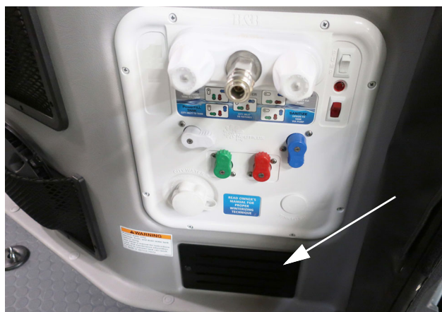
Water Pump (Located below Water Center Panel - remove panel to access) -Typical View
